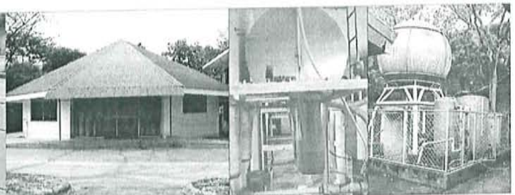
Water Filtration/ UV Light Treatment & Storage
